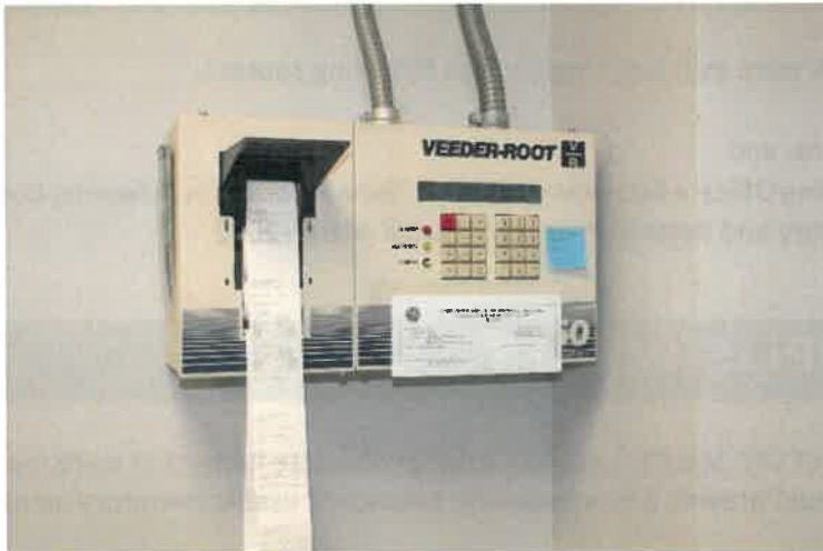
Public Works Fuel Veeder-Root Fuel Monitor
